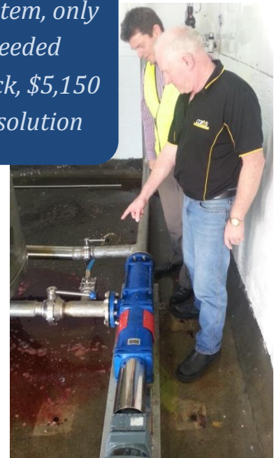
Blue Mono pump and 1,800 litre holding tank with level switch (above)
