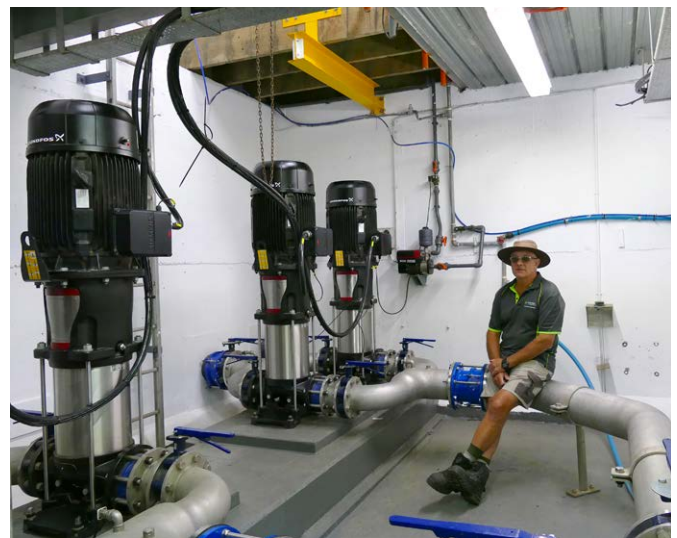
Figure 3: Whakatāne Team Leader Water Treatment Plant, Three Waters Operations Neal Yeates at the Braemar pump station.
